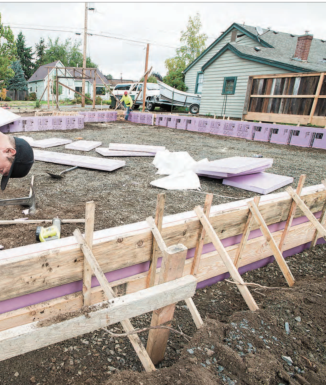
passive structure. Before concrete is poured inside the frame, crews will lay down six layers of 2-inch thick insulation to keep cold Debbie and John Pitney break a bottle of bubbly on the bucket of the excavator, signaling the start of construction. Submitted photo
